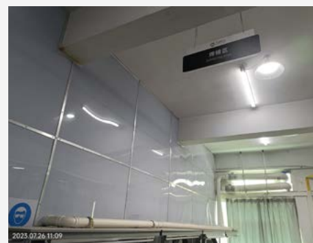
The air duct purification unit
