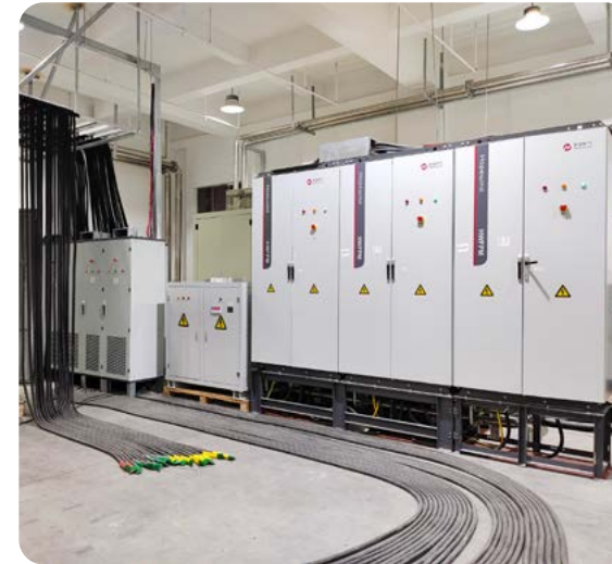
10 MW Wind Power Converter Standard Testing Platform
