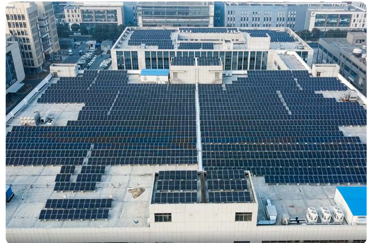
The distributed PVs in the Suzhou plant
