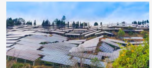
On-site image of 300MW Photovoltaic Composite Project in Lincang City, Yunnan Province
