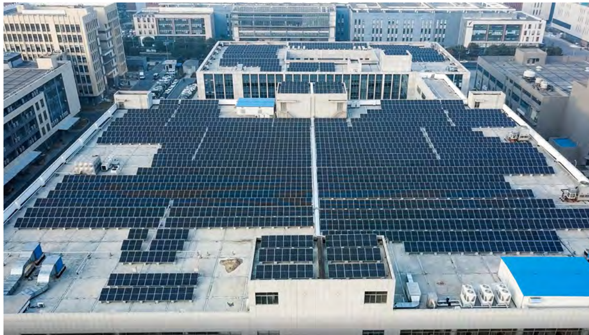
Hopewind's distributed rooftop photovoltaic systems
