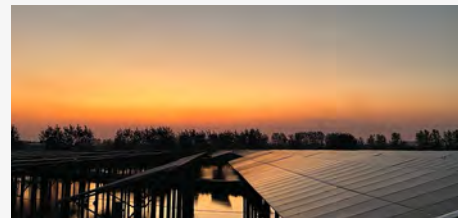
160MW Fishery-PV Complementary Project in Xishui, Hubei Province
