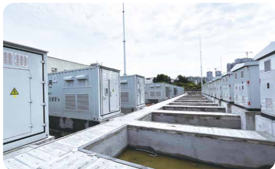
> 13MW/26MWh Grid-side energy storage project in Guangzhou, Guangdong
