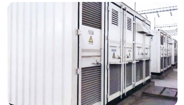
> Energy storage EMS project of a metal factory in Jiangyin City, Jiangsu Province
