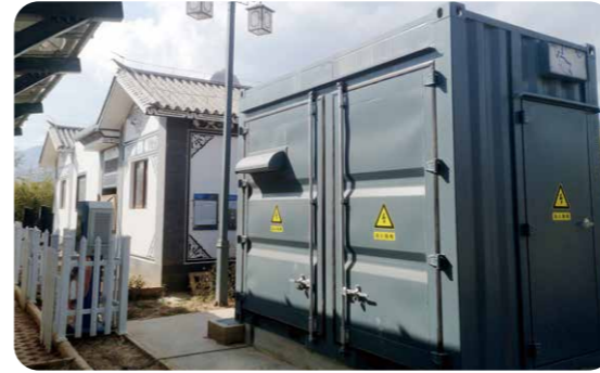
> Yunnan Microgrid Project
