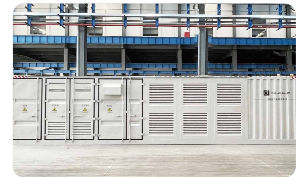
> 1MW Flywheel System Integration
