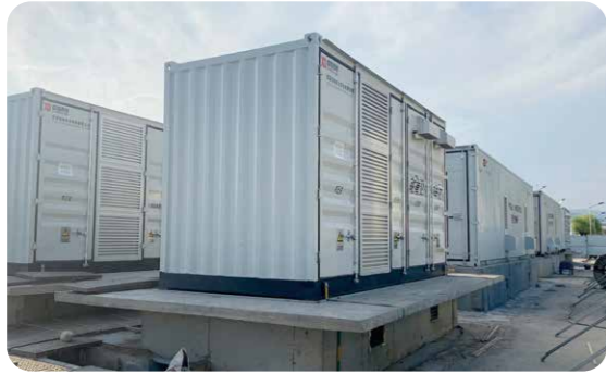
> 10MW/5MWh Thermal Power Plant Energy Storage Project in Hohhot, Inner Mongolia
