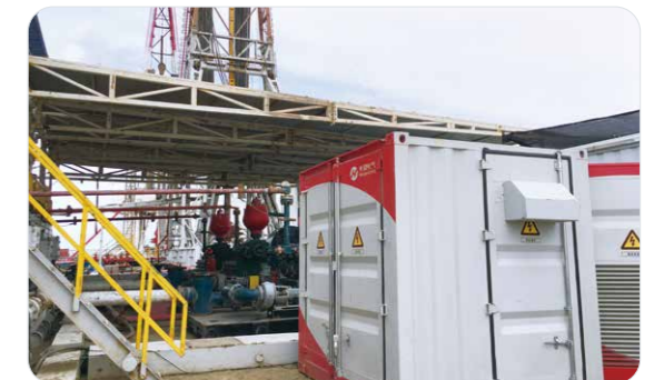
> Industrial energy storage project in Karamay city, Xinjiang autonomous region
