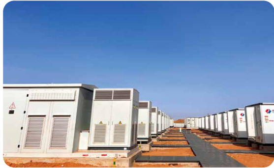
> 50MW/100MWh Independent energy storage project in Wuzhong city, Ningxia
