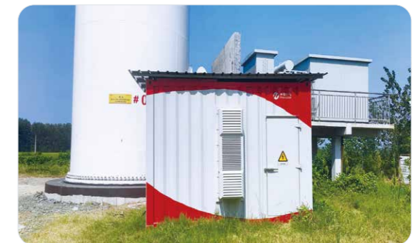
> Wind power DC-side energy storage project in Tianmen city, Hubei province
