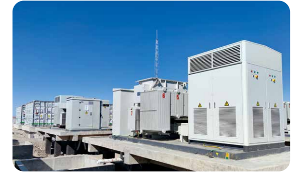
> 40MW/80MWh Generator-side energy storage project in Jiuquan city, Gansu province
