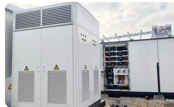
> 5MW/10MWh User-side energy storage project in Taizhou city, Zhejiang province
