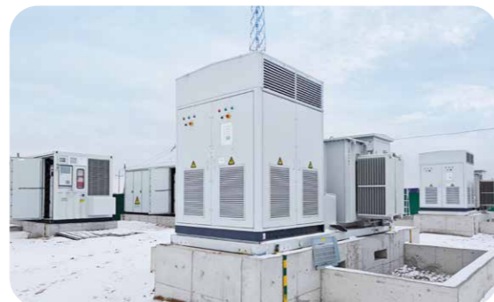
> 7.5MW/15MWh Generator-side energy storage project in Huhhot city, Inner Mongolia
