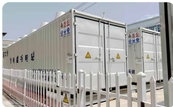
> 3MW/31MWh Energy Storage Power Station in Changxing, Zhejiang Province
