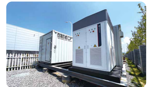
> 1.5MW/3MWh User-side energy storage project in Changxing county, Zhejiang province
