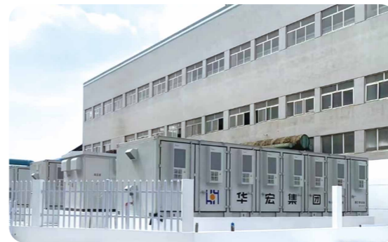
> Energy storage EMS project in Jiangyin City, Jiangsu Province
