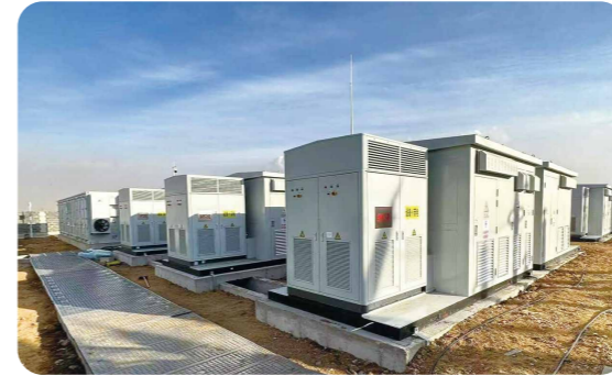
> 50MW/100MWh Generator-side energy storage project in Hulun Buir city, Inner Mongolia
