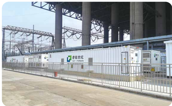
> 15MW/7.5MWh Thermal-energy Storage Frequency Modulation Project in a Power Plant in Shanxi Province
