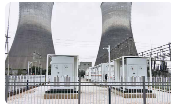
> 6MW/6MWh Coal-fired power station energy storage project in Chongqing city
