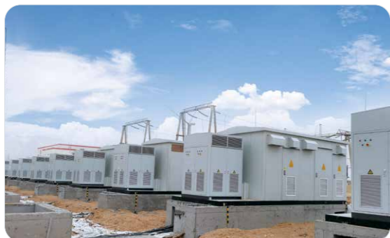
> 60MW/120MWh Generator-side energy storage project in Alxa League, Inner Mongolia
