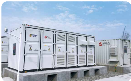
> 4MW/6MWh Generator-side energy storage project in Luohe city, Henan province
