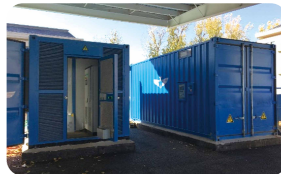
> Micro-grid EMS project in Fangshan District, Beijing
