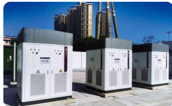
> 6.25MW/12.5MWh Grid-side energy storage project in Guangzhou, Guangdong
